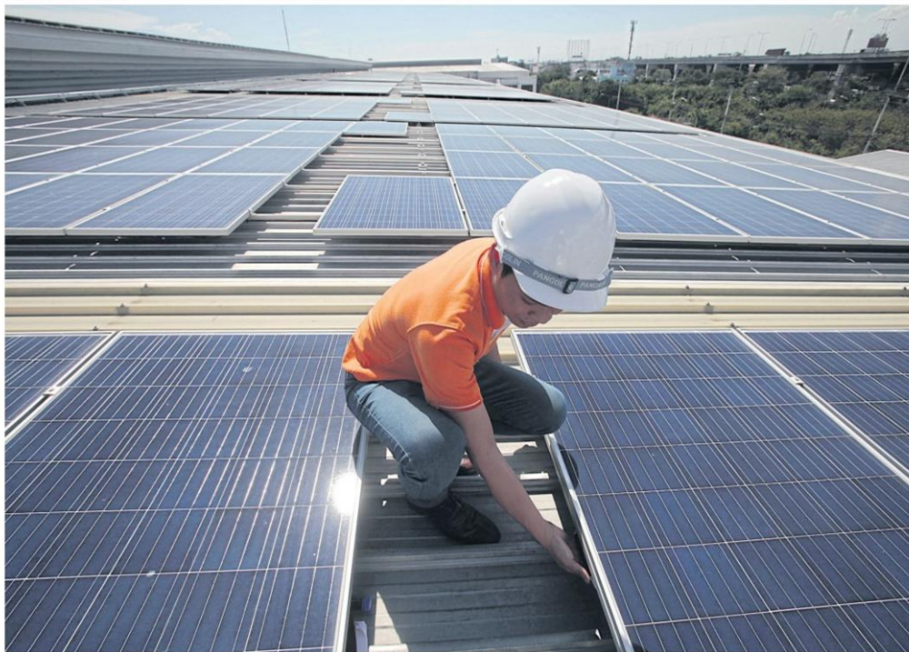
A worker installs solar panels in Samut Prakan. Gunkul has a partnership with WHA Corporation Plc on the project. PORNPROM SATRABHAYA
